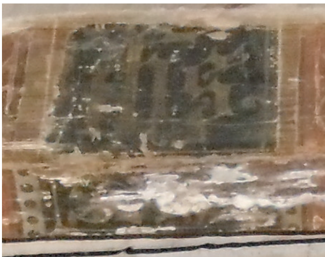
Fig. 10 Detail of one of the supporting beams of the bell wheel of Petra bearing the IHS monogram. This is the only instrument featuring extant inscriptions. Photo by the author.
