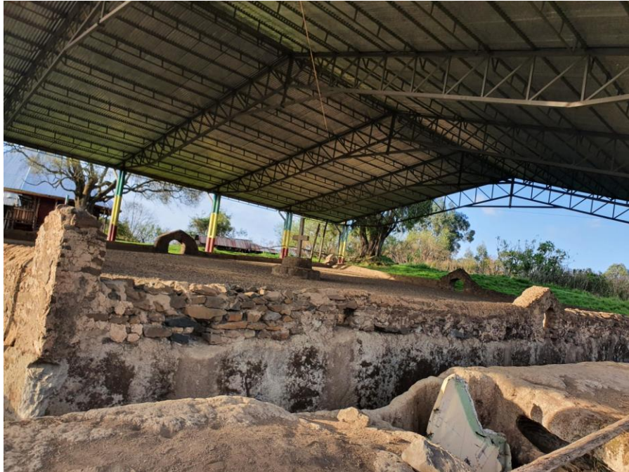
Figure 4. The masonry over the roof's edge of the rock-hewn church. Source: author (2021).
